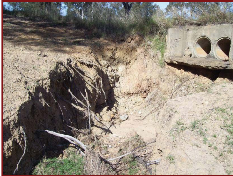
Photo 13 – Localised erosion scour in the north eastern portion of the site (note dam overflow culvert)
